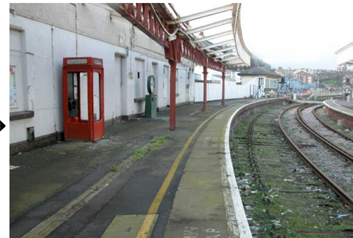
Falling into disrepair.
