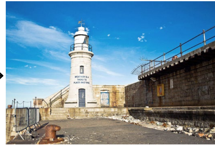
Falling into disrepair.
